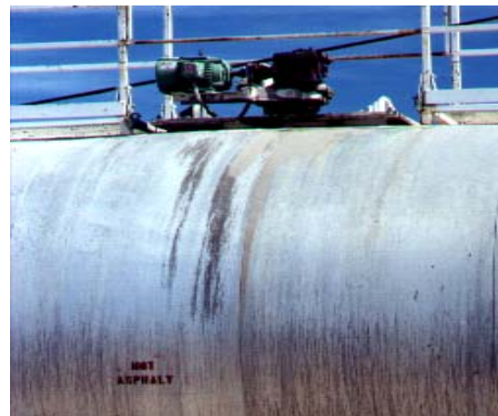
Figure 3-3: Auger For Agitating Asphalt Rubber Storage Tank
